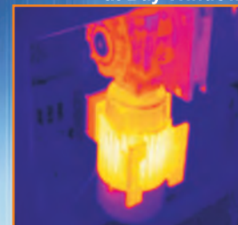
Overheating Drive Thermograph
